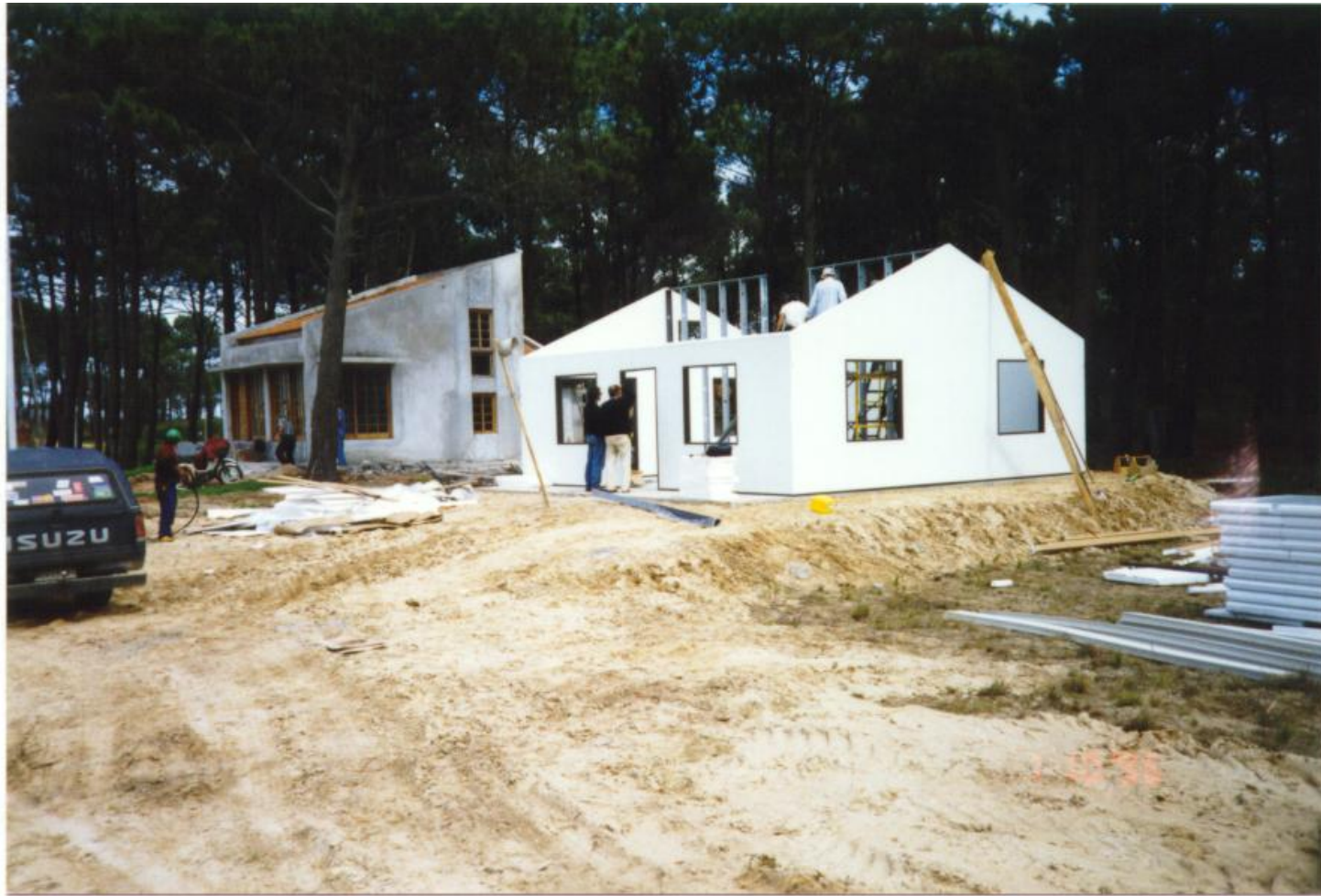
Hour 6 - View of completed exterior wall panels ready for roof panel installation.
