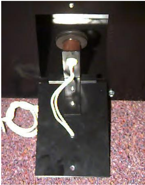
Photo shows float panel opened up with the optional automation float installed. Note: the float wires are routed through the opening on the panel to the front.
